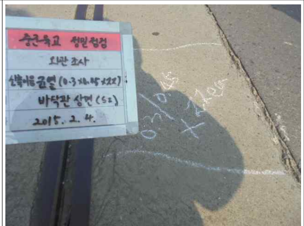
A2 Rail Joint 후타재 균열
